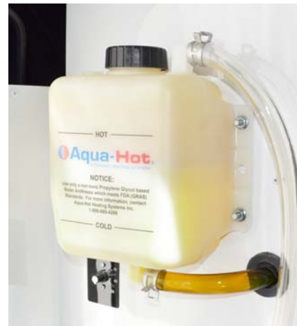
Expansion Fill Tank
