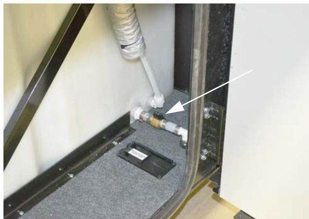
Water Tank Drain Valve (Located in the third passenger side compartment) -Typical View
