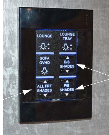
12-Volt Night Shade Switches - Lounge *Switch located by sofa shown -Typical View
