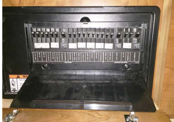
House Circuit Breakers -Typical View
