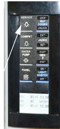
(Located in water service center) - Typical View
