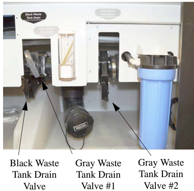
Black and Gray Waste Tank Drain Valves (Located in water service center)
