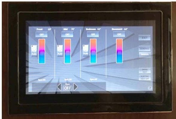
Basement Temperature Control (Located on touch tablet)
