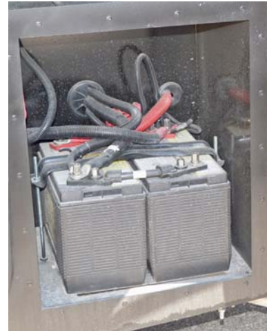
Chassis Batteries (Located behind a rear driver side exterior door) -Typical View
