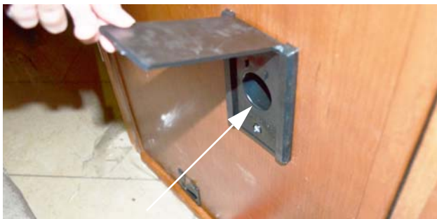
Interior Hose Outlet
