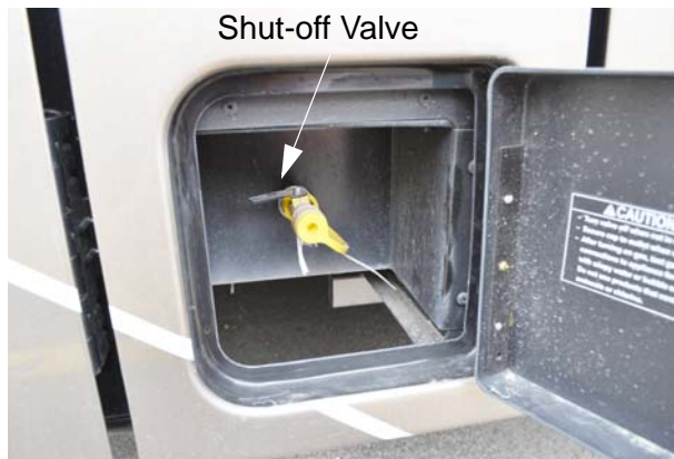
LP Accessory Connection (Located behind lockable access door on passenger side of coach) -Typical View
