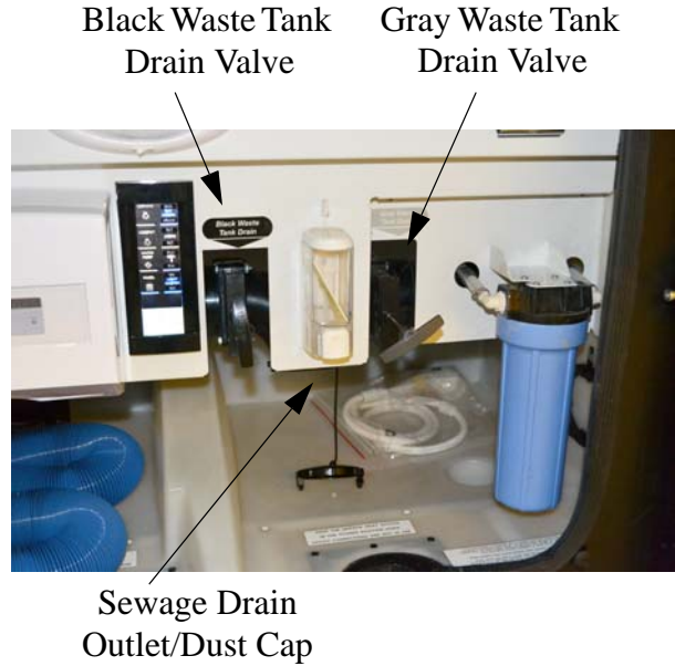
Black and Gray Waste Tank Drain Valves (Located in water service center)
