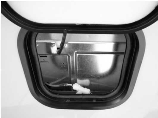
Residential Refrigerator Service Compartment (Located along driver or passenger sidewall, depending on model) -Typical View
