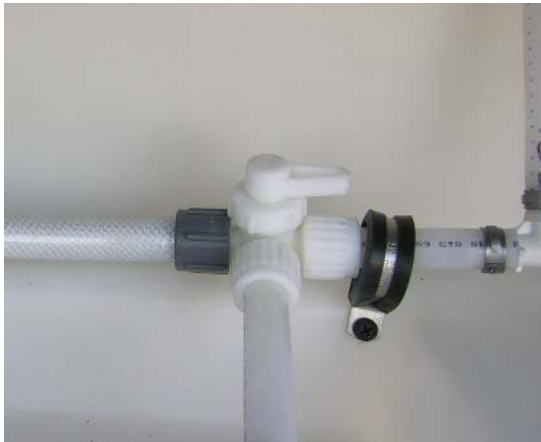
Waterline Drain Valve -Typical installation shown
