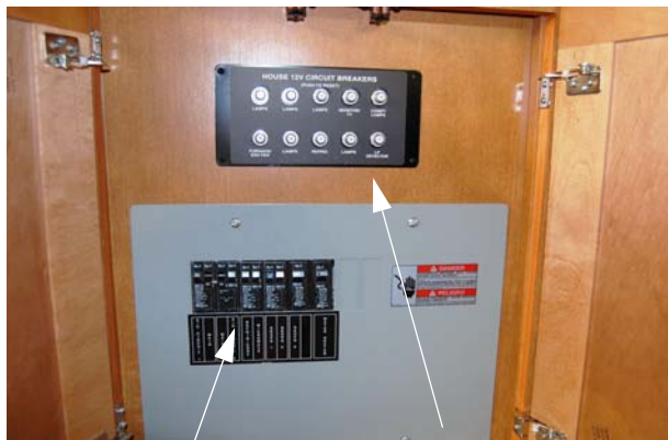
120-Volt House Circuit Breakers
