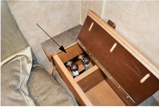
Water Supply Faucets (Located inside front nightstand)
