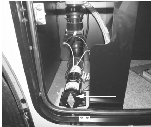
Waste Pump (Located in passenger side compartment ahead of rear axle) -Typical installation shown
