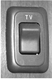
Bedroom TV 12-Volt Master Power Switch (Located on cabinet or wall near TV) -Typical installation shown
