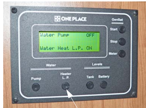
LP Gas Water Heater Switch
