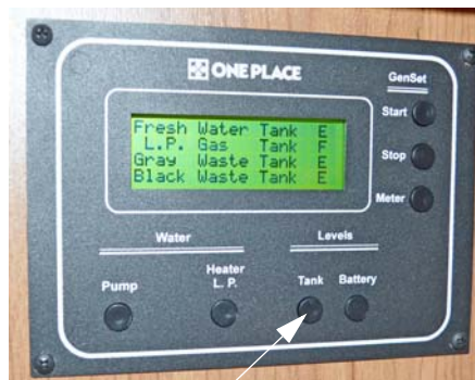
Tank Levels Switch
