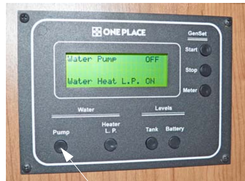
Water Pump Switch
