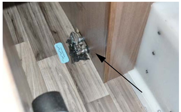
Waterline Drain Valve
