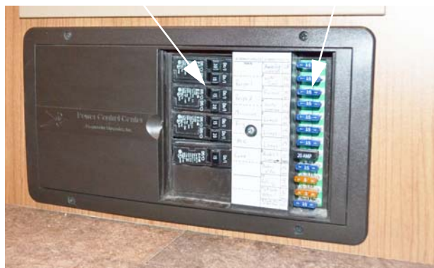
Power Center (Converter) -Typical View
