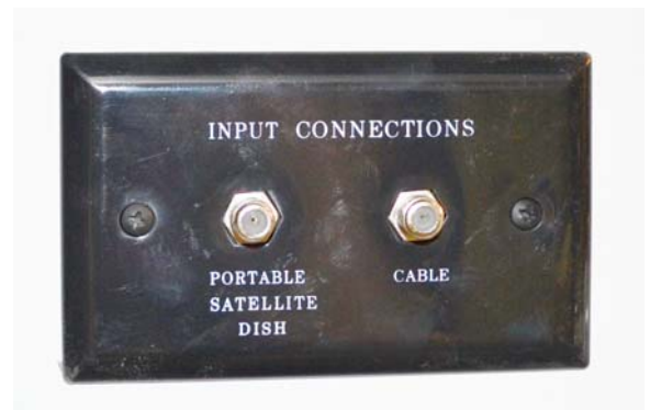
Cable TV and Satellite Connections (Located in shoreline compartment)
