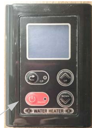
Water Heater Power Switch (Push to turn ON)
