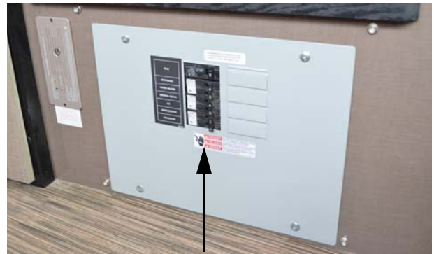
120-Volt Circuit Breakers -Typical View
