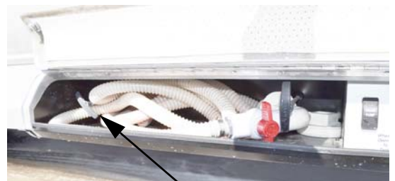
Gray Waste Tank Drain Valve (Located in water service center)
