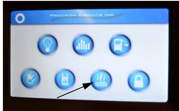
Water Pump Switch
