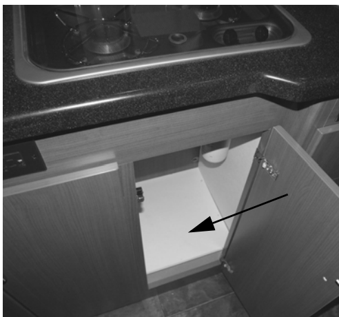
Water Pump (Located beneath removable panel under galley)
