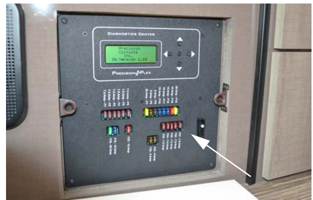
House 12-Volt Fuses -Typical View
