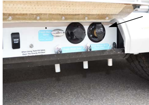
Black Waste Tank Flush Inlet (Located in water center compartment) -Typical View
