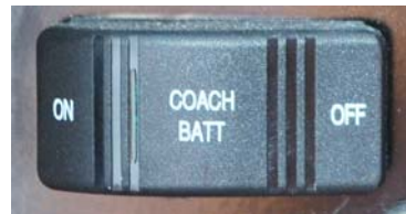
House/Coach Battery Disconnect Switch
