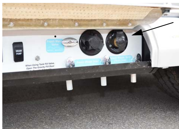
Black Waste Tank Flush Inlet (Located in water center compartment on the driver side of motorhome) -Typical View
