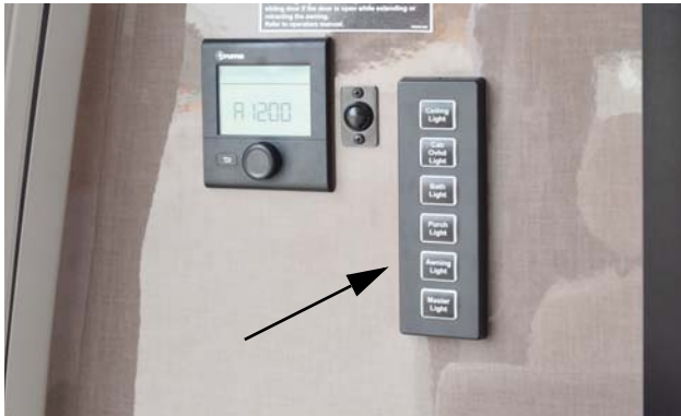
Awning Light Switch (Located near monitor panel or front of galley, depending on model) -Typical View
