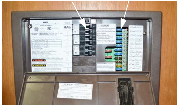
Power Center (Converter) -Typical View
