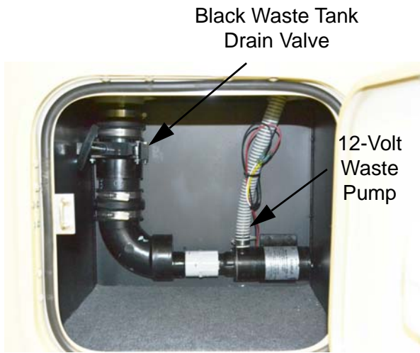
Black Holding Tank Waste Pump (Model 27PE Only - Located inside a passenger compartment)
