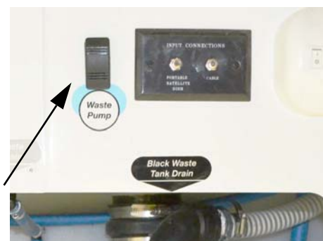
Waste Pump (Located in water service center on driver side of coach)
