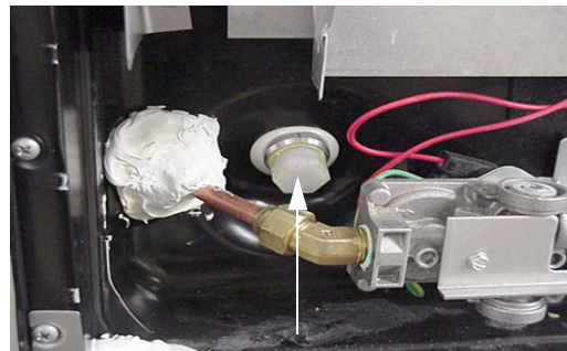
Water Heater Drain Plug (Remove with socket)
