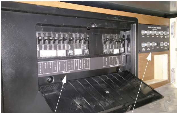
120-Volt House Circuit Breakers
