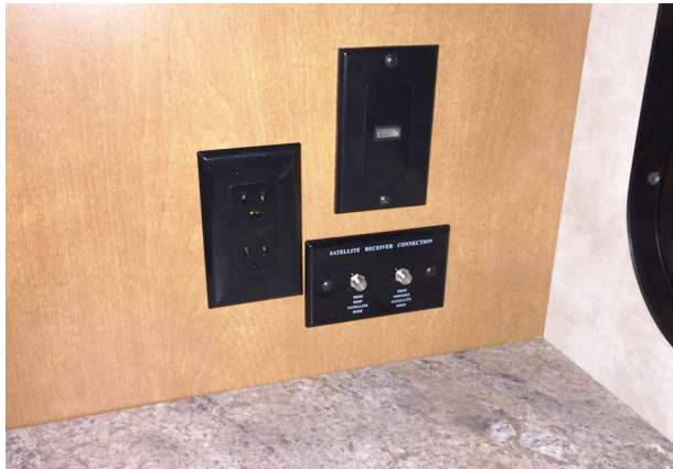
Bedroom DVD/Satellite Receiver Connection -Typical View
