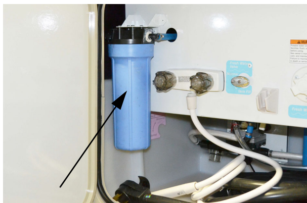
Full-Coach Water Filter System (Located in water service center) -Typical View
