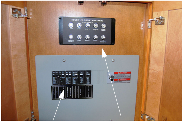
120-Volt House Circuit Breakers
