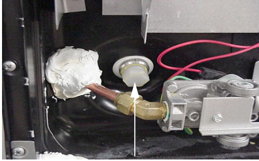
Water Heater Drain Plug (Remove with socket)
