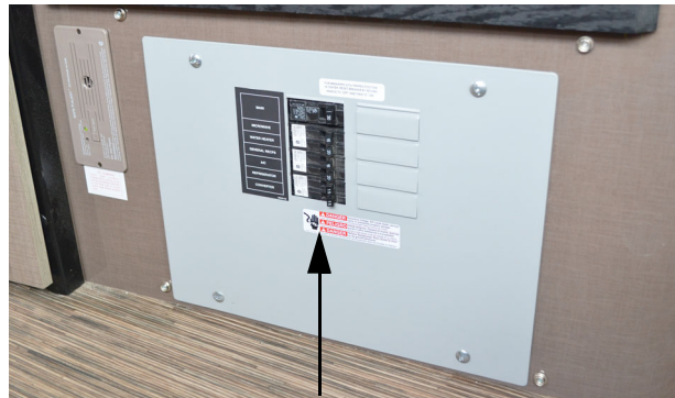
120-Volt Circuit Breakers -Typical View
