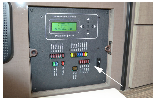
House 12-Volt Fuses -Typical View
