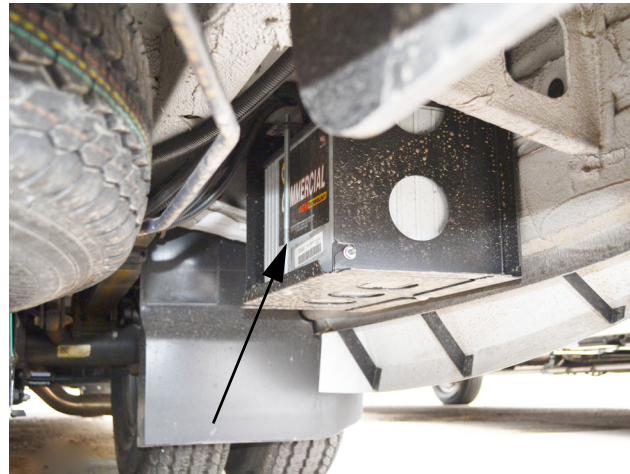
House Battery Access
