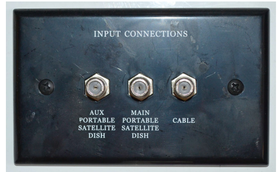
Satellite Dish and Cable TV Connections (Located in utility compartment, shoreline compartment, or water service center, depending on model) -Typical View
