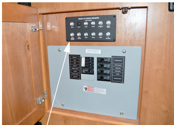
House 12-Volt Circuit Breakers
