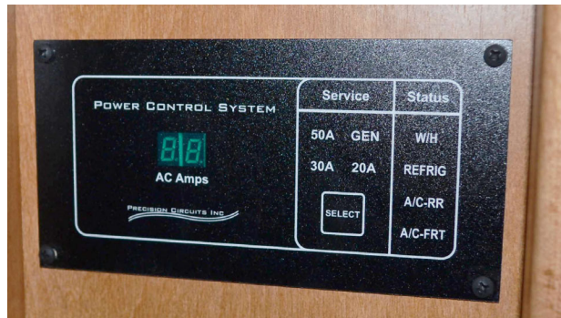
PCS Display Panel (Located near monitor panel) -Typical View
