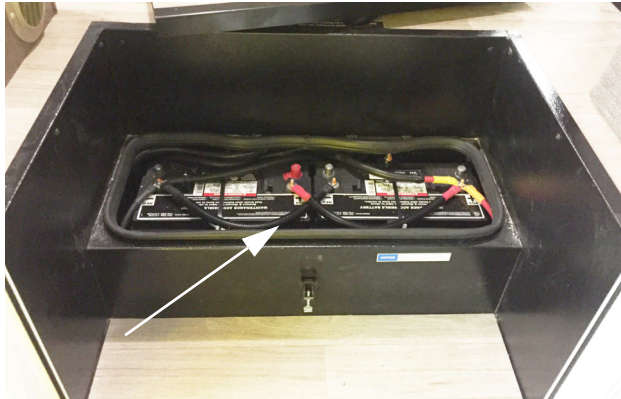
House Batteries (Entrance Step Removed) -Typical View
