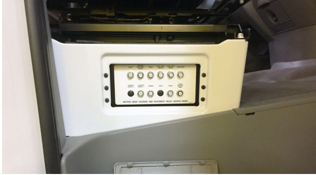
Automotive Chassis 12-Volt Circuit Breakers (Located on outboard side of passenger seat) * Shown with cover removed -Typical View
