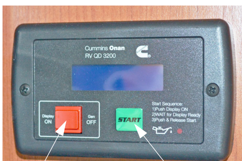
Press to Stop/Prime Press to Start Diesel Generator Start/Stop Buttons (Located near monitor panel) -Typical View
