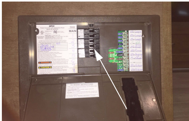
120-Volt Circuit Breakers -Typical View
