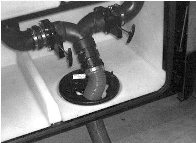
Drainage Hose routed through passage in compartment
