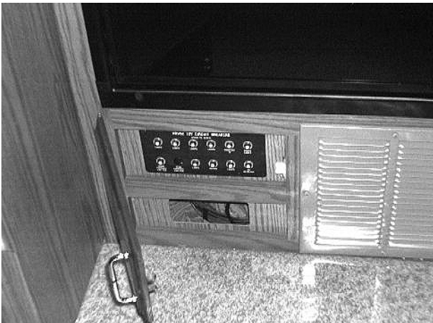
House 12V Breakers (below refrigerator)
