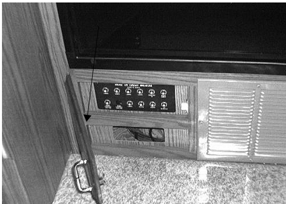
House 12-Volt Circuit Breaker Panel
