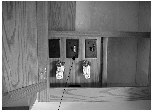
Water Heater Switch Electric Operation
