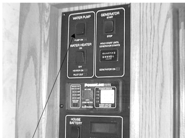
Water Pump Switch
