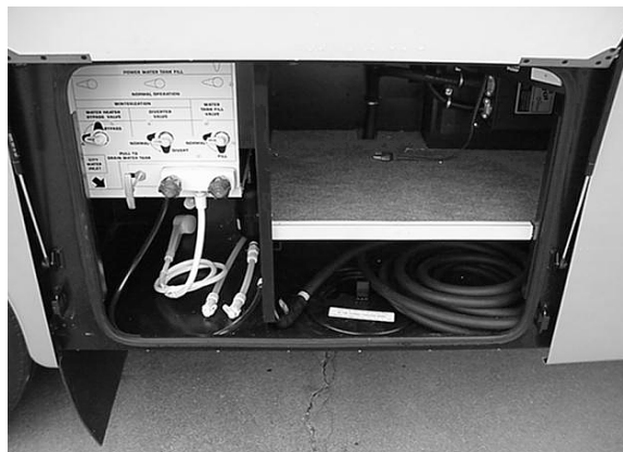
Water Center/Shoreline Compartment
