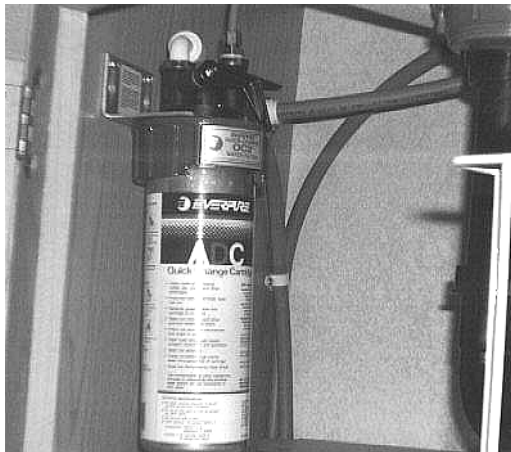
Water Filter Assembly - Below Galley Sink
