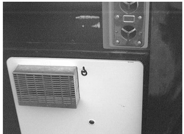
Water Heater Service Access Panel
