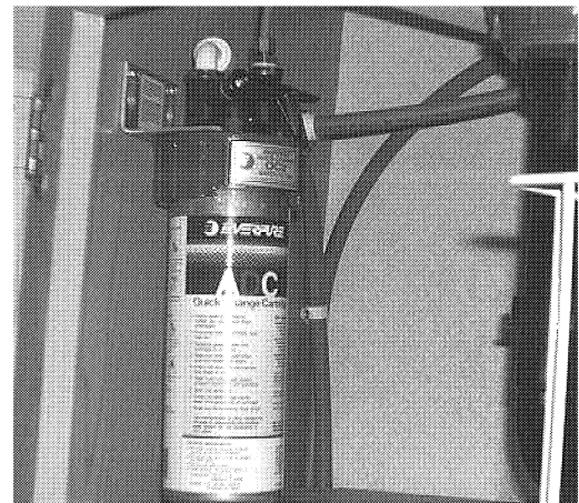
Water Filter Assembly - Below Galley Sink
