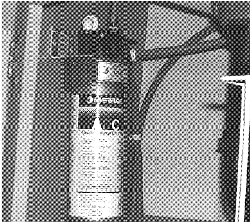
Water Filter Assembly - Below Galley Sink
