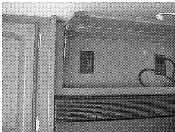
Electric Water Heater Switch (above microwave)
