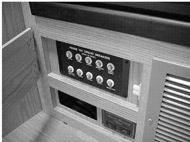
House 12-Volt Breaker Panel
