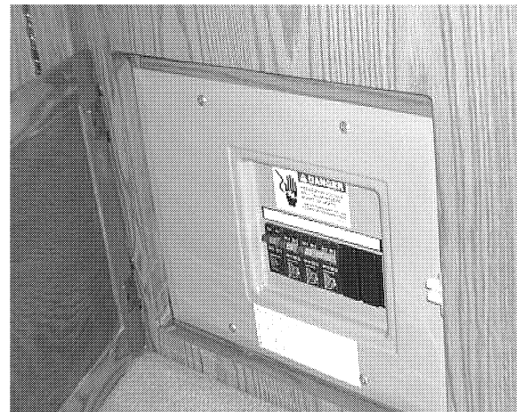
House 110-Volt Breaker Panel near Entrance Step
