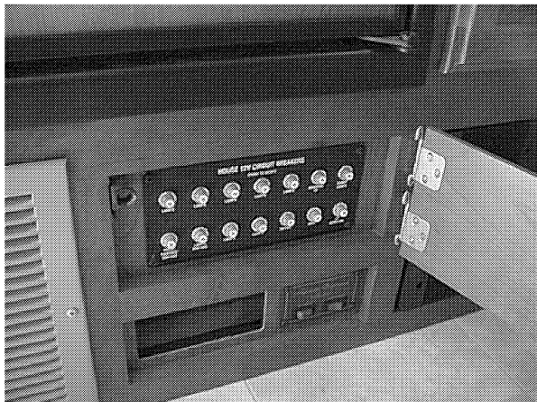
House 12-Volt Breaker Panel
