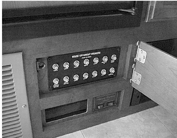
House 12-Volt Breakers
