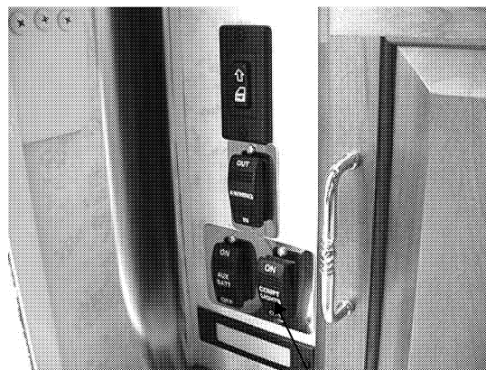
Compartment Lights Switch
