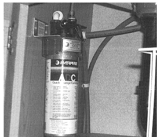
Water Filter Assembly - Below Galley Sink
