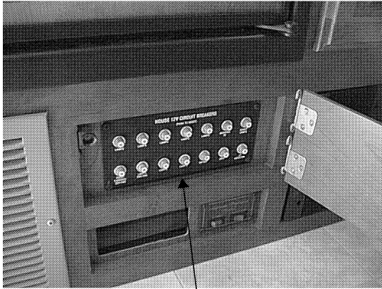
House 12V Breakers
