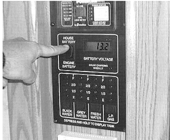
Battery Voltage Check One Place Panel
