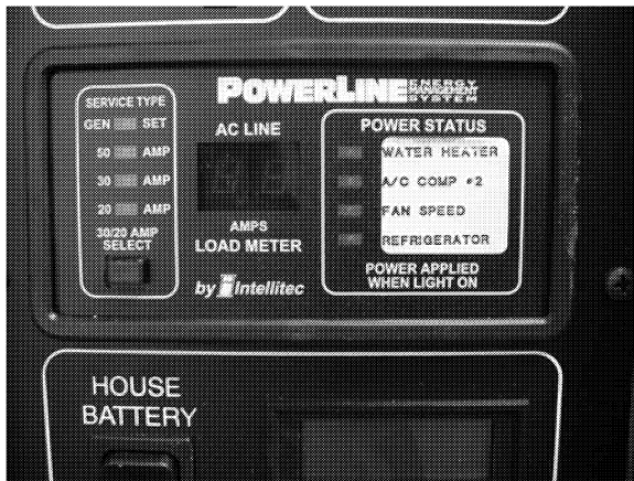
EMS Display on OnePlace Monitor Panel
