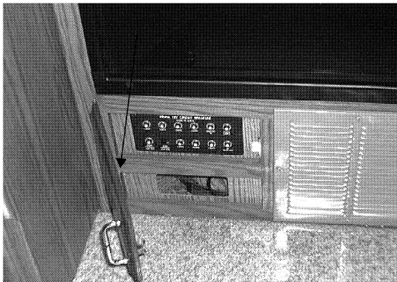
House 12-Volt Circuit Breaker Panel
