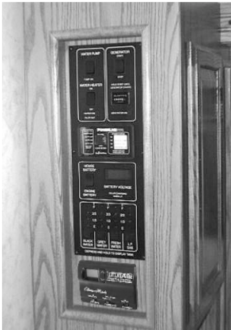
One Place Monitor Panel
