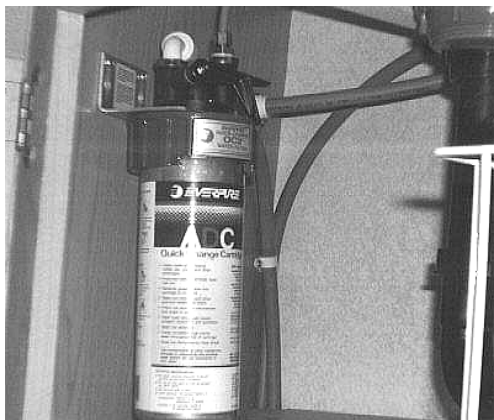
Water Filter Assembly - Below Galley Sink
