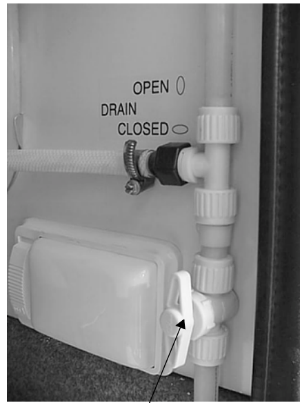
Water Line Drain Valve
