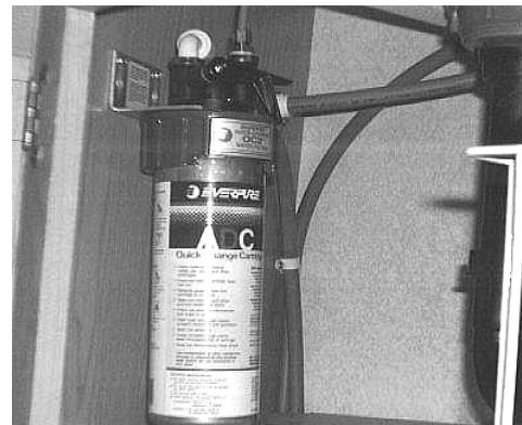
Water Filter Assembly below Galley Sink
