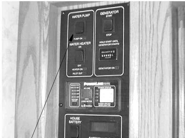
Water Pump Switch
