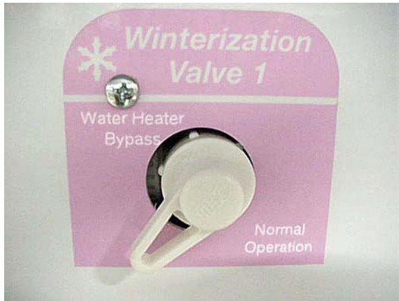
Water Heater Bypass Valve
