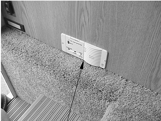
LP Gas Leak Detector
