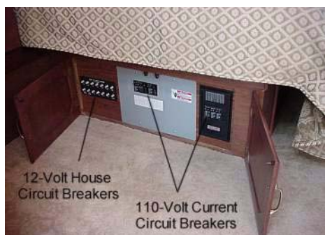
House 12V Breakers
