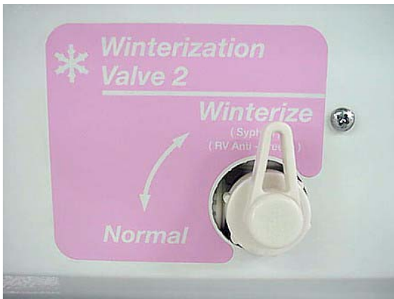
Winterization Valve in water service center
