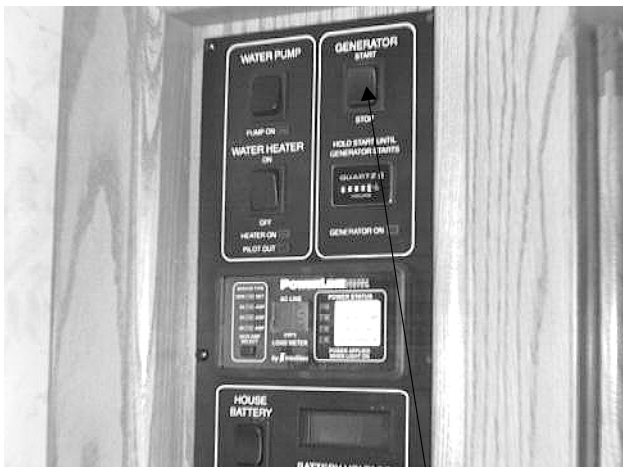
Generator Switch and Hourmeter
