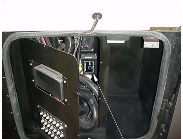
Keyless Entry Control Box in 12-volt electrical compartment.
