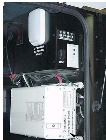
Inverter Charger Unit Location in utility compartment
