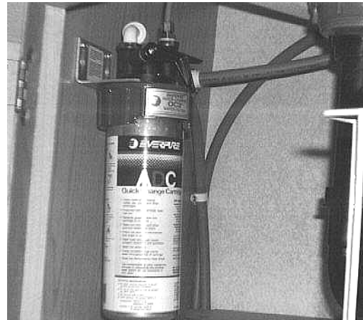
Water Filter Assembly below galley sink
