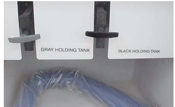
Holding Tank Valves in Water Service Center
