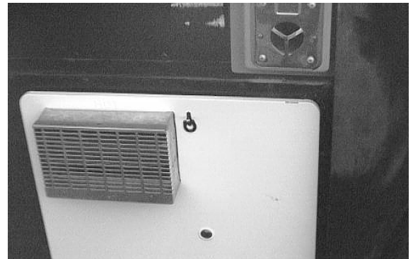
Water Heater Exterior Service Access
