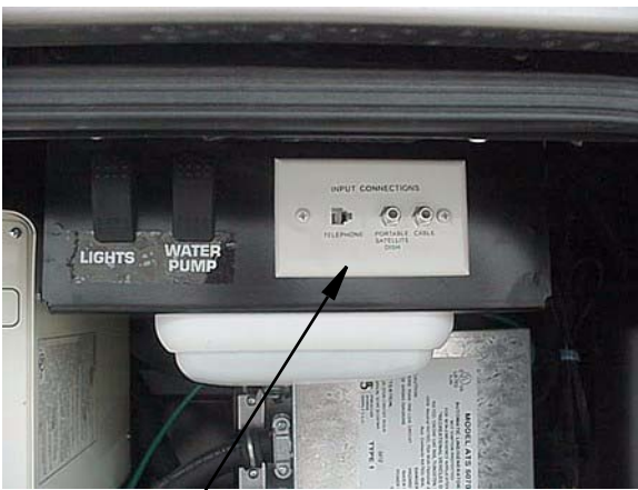
Exterior Input Connections for Satellite Dish, Cable TV and Phone (in Water Center or Shoreline Compartment)
