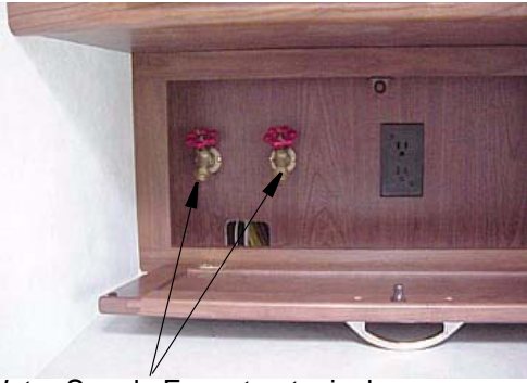
Water Supply Faucets - typical
