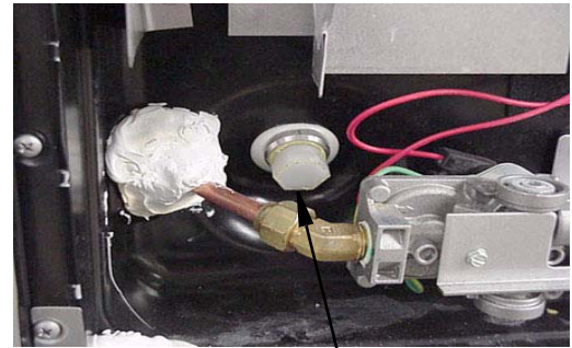
Water Heater Drain Plug Remove with socket.
