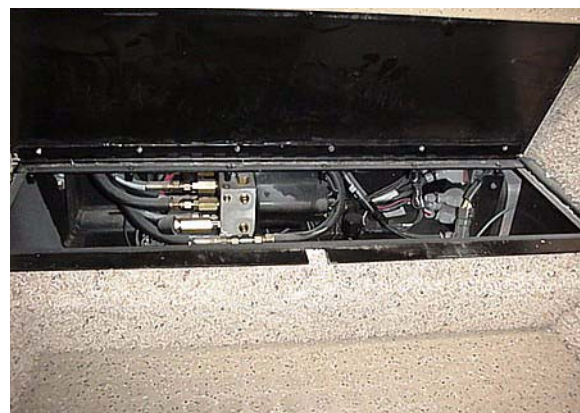
Hydraulic Pump beneath Entry Step
