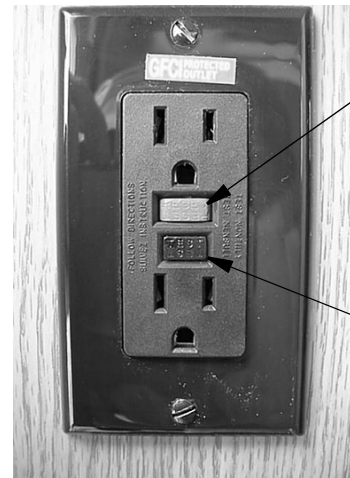
GFCI Outlet (Ground Fault Protector)
