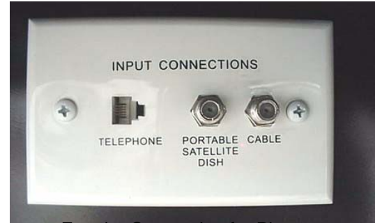
Exterior Connection for Phone, Satellite Dishes and Cable TV (In Water Center or Shoreline Compartment)
