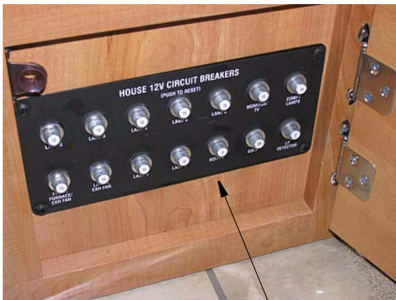
House 12-Volt Circuit Breaker Panel
