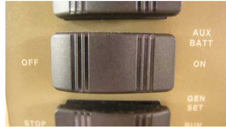
Aux. Battery Switch (on dash)
