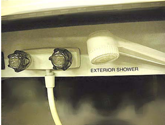
Exterior Shower/Wash Station (Typical)
