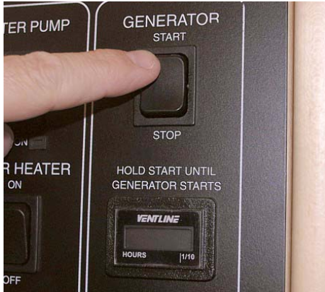
Generator Switch and Hourmeter on monitor panel
