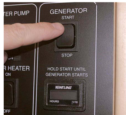
Generator Switch and Hourmeter
