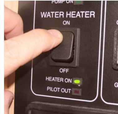
Gas Water Heater Switch (on Systems Monitor Panel)
