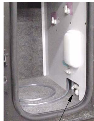
Waterline Drain Valve
