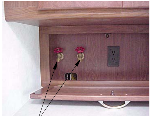
Water Supply Faucets - Typical View
