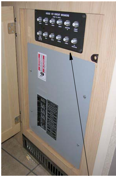
House 12-Volt Circuit Breaker Panel
