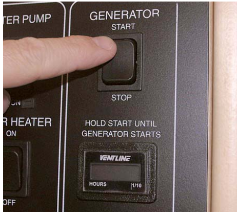
Generator Switch and Hourmeter on monitor panel
