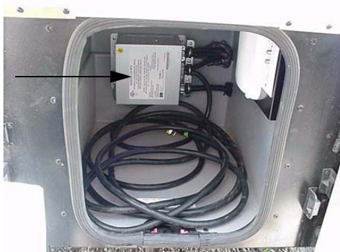
Power Transfer Switch Box (Typical View)
