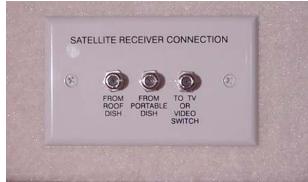
Interior Connection for Satellite Dishes (Located in cabinet near TV) - Typical View
